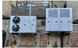
The units which have been attached to the rear of a High Street premises
